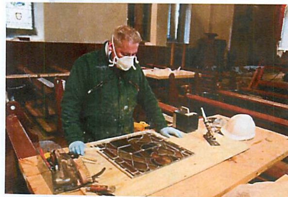
A workman refurbishes a panel of glass inside St Magnus Church as the restoration was progressing. Not all the windows could be dealt with on site and so many were take to Glasgow for re-leading at the Cannon MacInnes workshop [picture Cannon MacInnes]
